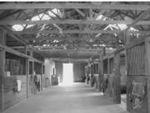
Figure 3.2. Clear-span construction uses wooden arches that provide an open interior. Stall corner posts attach to the lower chord of some trusses but are not supporting the roof weight.
